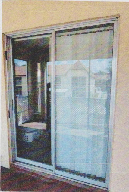
Unprotected glazed entry door
