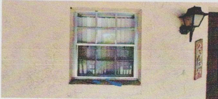
Unprotected glazed opening
