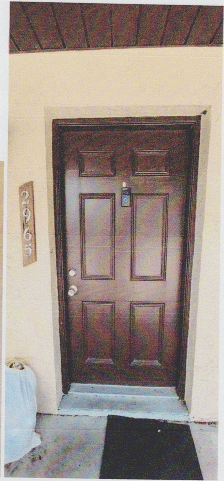
Unprotected non-glazed entry door
